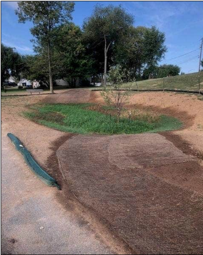
Project 7 rain garden at Anderson Park post-construction
